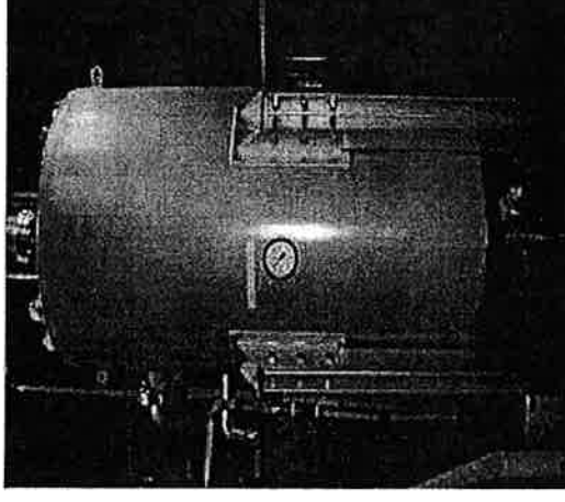
Cooling water circulation tank
